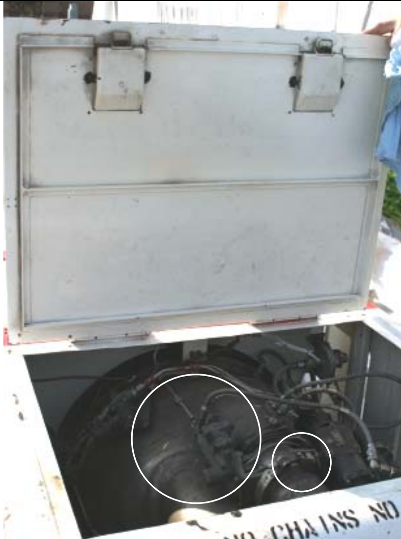
Figure 5 –Circled areas highlight typical heat vent source areas on the A/S47A-1 Enclosure panel
