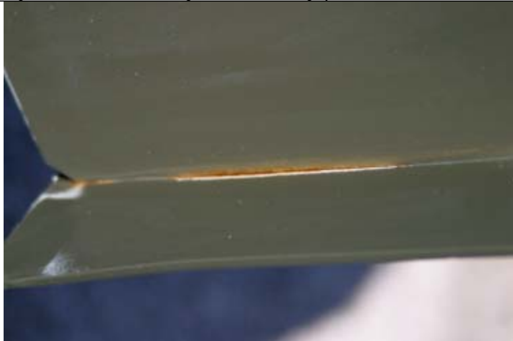
Figure 9 – Typical induced coating defect after 18-months exposure at Cape Canaveral AFS, FL
